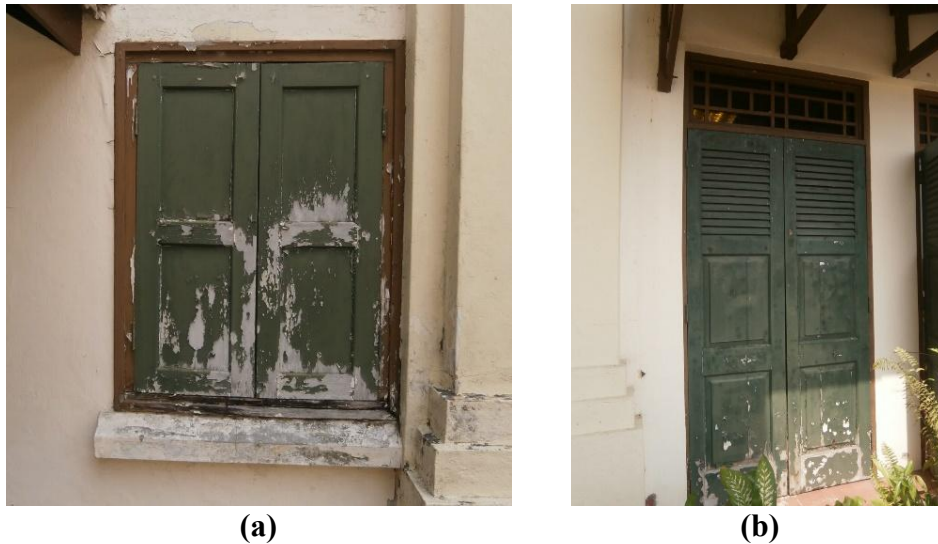
Figure 7. Peeling paint condition on: (a) window and (b) door Source: Individual Analysis, (2025).
