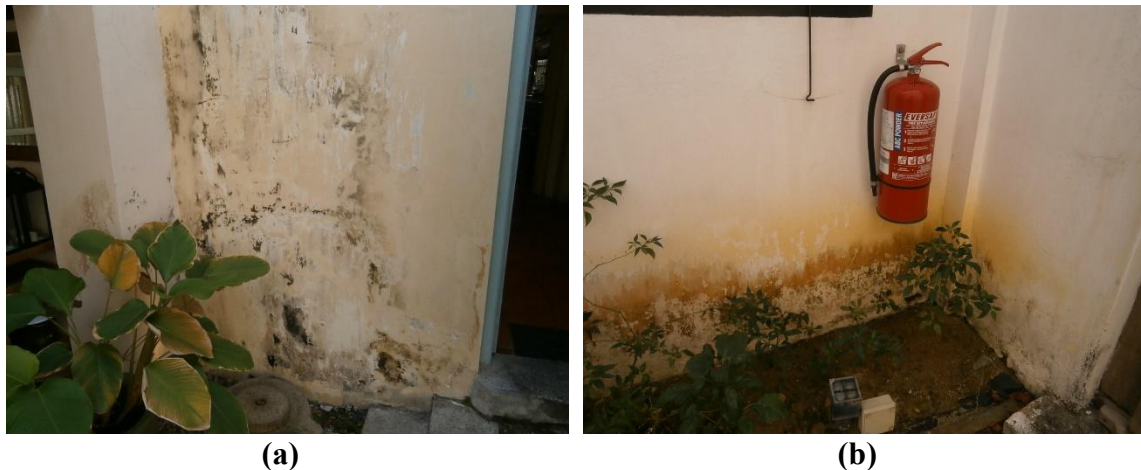
Figure 3. Fungi/mold visible on outside of building:(a) near Indian Shophouse and (b) part of Jack annex roof Source: Individual Analysis, (2025).
